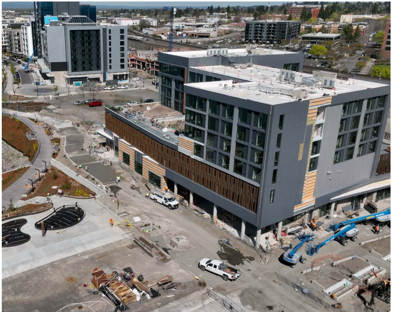
Final touches being made to AC Hotel by Marriott and Vancouver Landing, both scheduled to open this summer.
